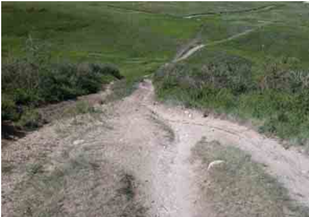
Figure 9.10 Steep Trails Cause Erosion of the Slope
