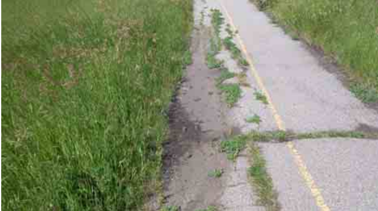
Figure 2.5 Current asphalt pathway is in poor disrepair
