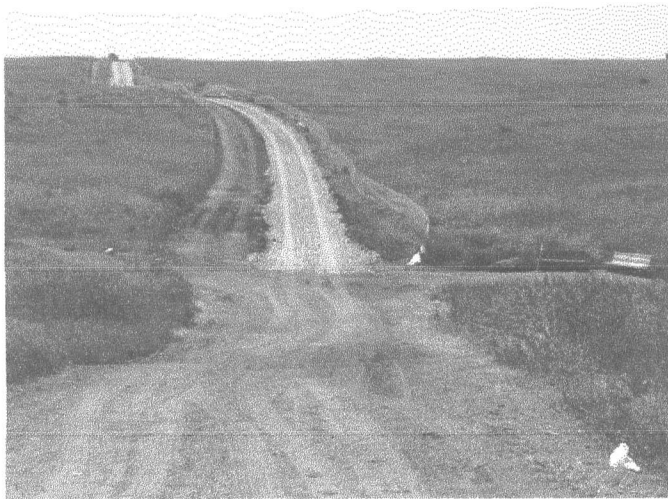
Sub-grade preparation: North end of north-south pathway (at intersection with existing chip-seal pathway)
