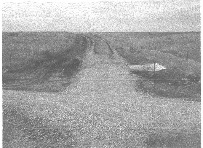
Asphalt base completed: North end of north-south pathway (at intersection with existing chip-seal pathway)
